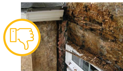
IMPROPERLY FLASHED DOOR HAS STRUCTURAL DAMAGE DUE TO WATER PENETRATION
