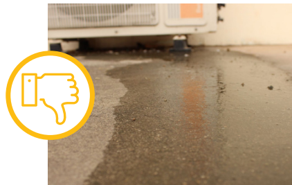
CONDENSATE DIRECTLY LEAKS ONTO A WALKWAY
