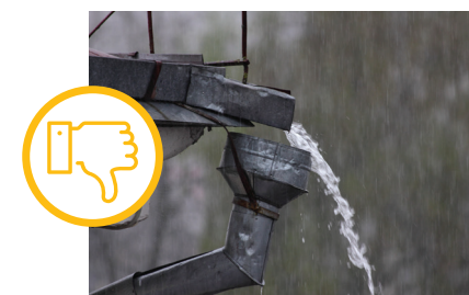
RUSTING, DISCONNECTED DOWNSPOUT
