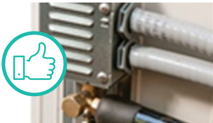
ALL LINE SET/REFRIGERANT LINES PROPERLY INSULATED Courtesy of PTCS
