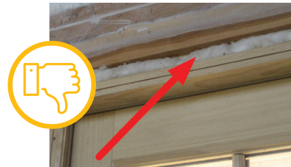
LOOSE-FILL INSULATION ALLOWS MOISTURE AND AIR INFILTRATION
