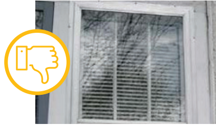
SINGLE-PANED ALUMINUM WINDOW WITH NO STORM OR LOW-E PROTECTION
