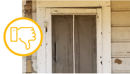
INEFFICIENT DOOR NEEDS TO BE REPLACED
