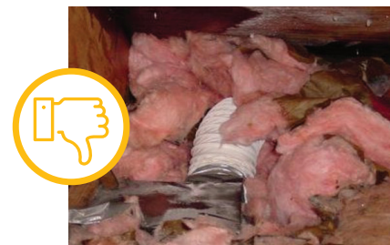
INTERIOR MOISTURE SOURCE NOT CORRECTED. THIS PROBLEM IS DUE TO AN UNVENTED FAN
