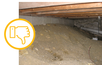
MISSING GROUND COVER
