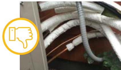
LINE SET/REFRIGERANT LINES NOT COMPLETELY INSULATED Courtesy of NW Ductless Heat Pump Project
