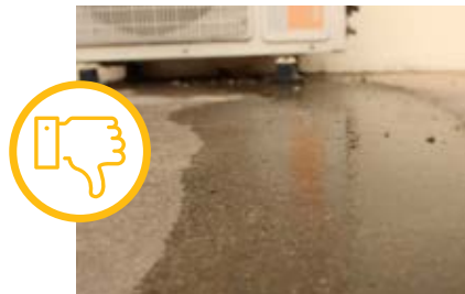
CONDENSATE DIRECTLY LEAKS ONTO A WALKWAY
