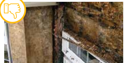
Improperly flashed door has structural damage due to water penetration. Courtesy of U.S. Department of Energy
