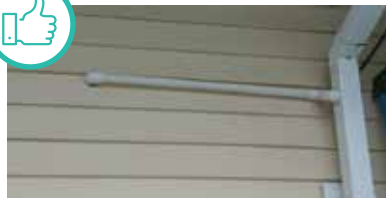
Condensate drain is connected to downspout.
