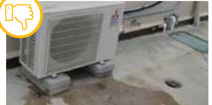
Condensate directly leaks onto a walkway.
